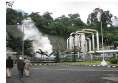
Geothermal Power Plants
